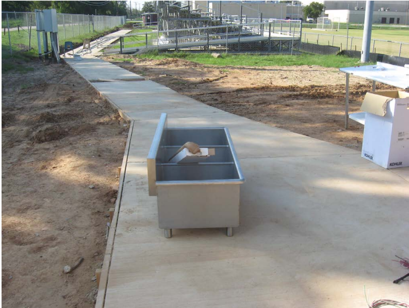
Stainless Steel Sink ready for installation in Concessions Building New Concrete Sidewalk from Concessions to Soccer Bleachers
