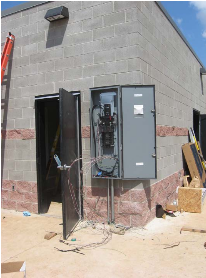
Concessions Building Electrical Service Panel
