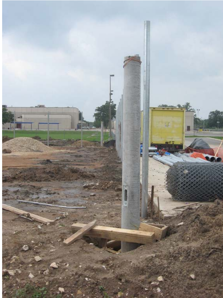
Tennis Court Lighting Support
