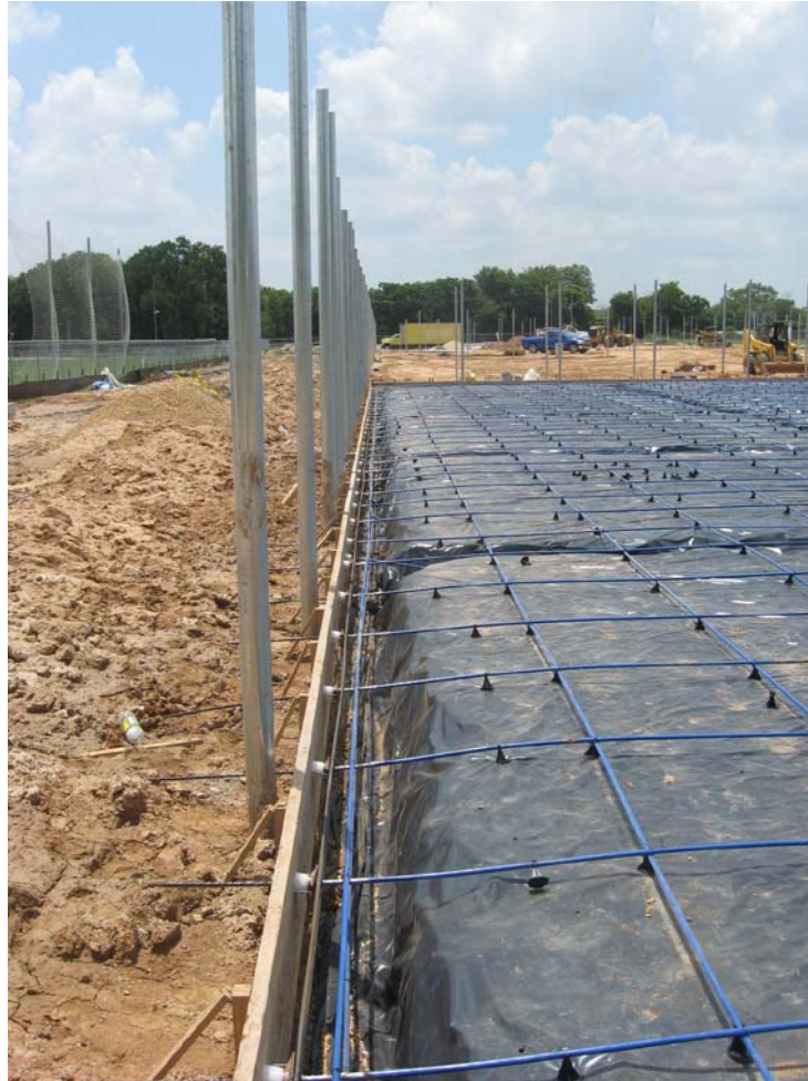
Tennis Court Fence Posts w/ Post Tension West View at North Soccer Fence
