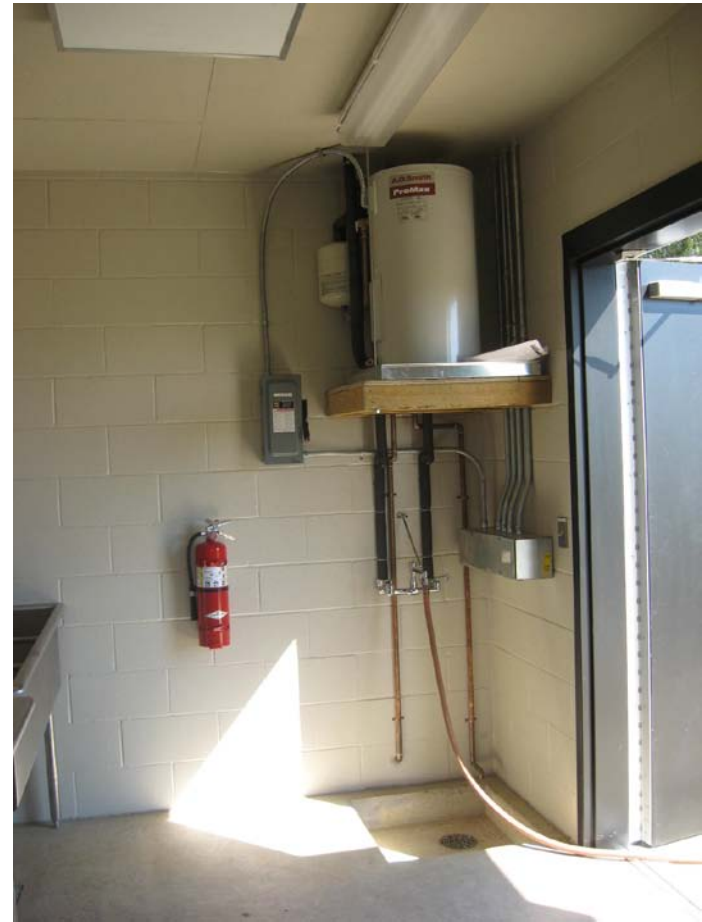
Interior Concessions Water Heater and Mop Sink
