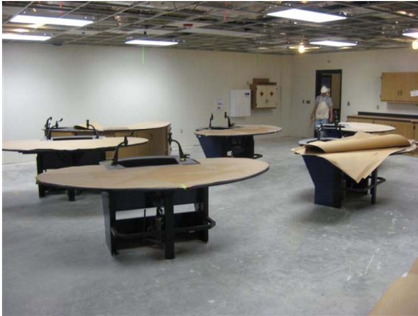
Science Desk Installation
