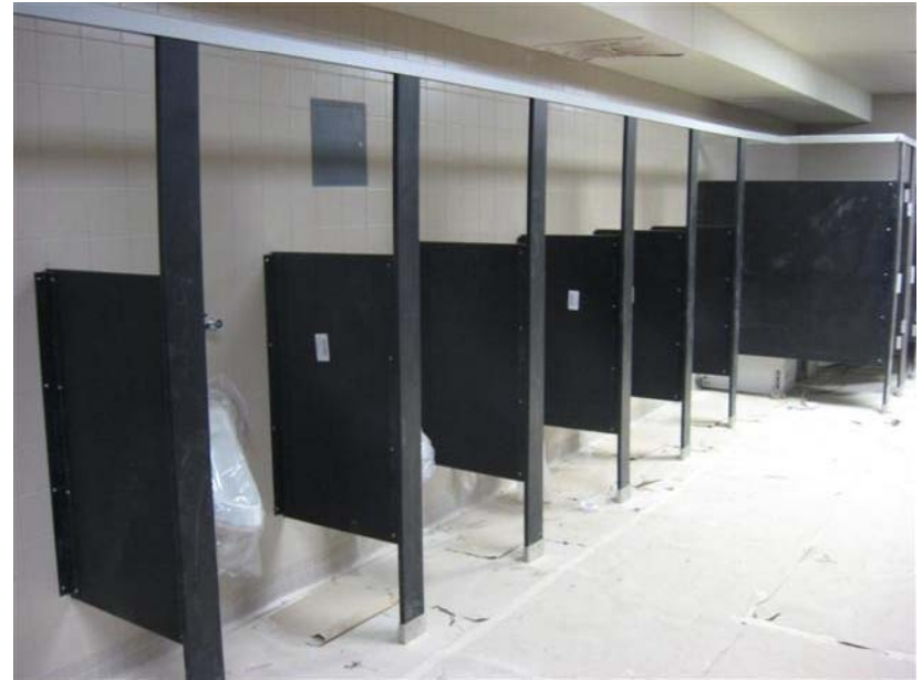
Toilet Partitions/ Fixtures at Restrooms
